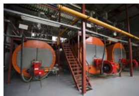
Boilers & Process Heat
