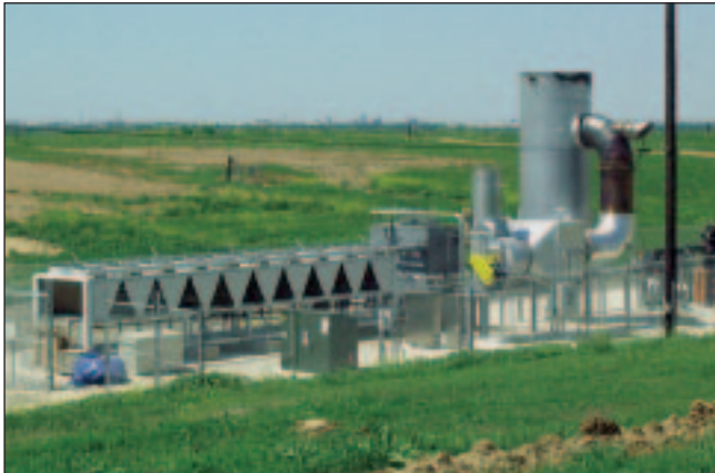
Landfill Flare Exhaust
