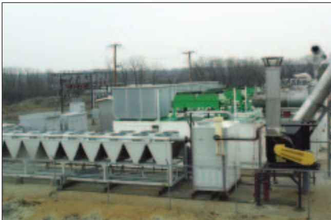
Reciprocating Engine Exhaust
